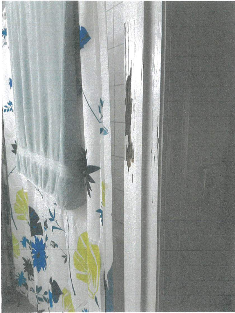
Bathroom door frame damaged by Termites
